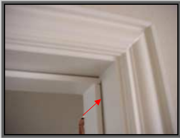
Weather-strip missing on door
