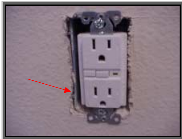
Envelope penetration not sealed
