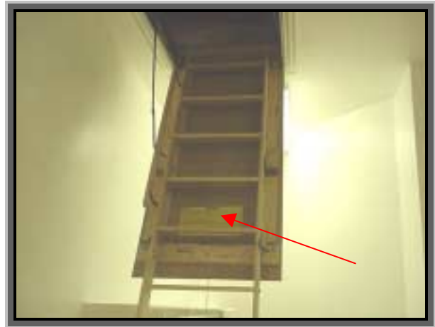
Attic access not insulated nor weather-stripped.
