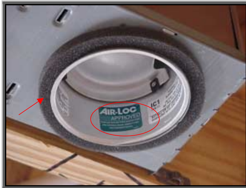
Properly labeled recessed can light with Gasket installed.
