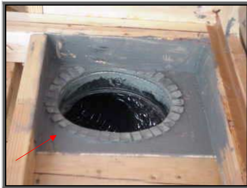
Mastic correctly installed at return air duct connection in wall
