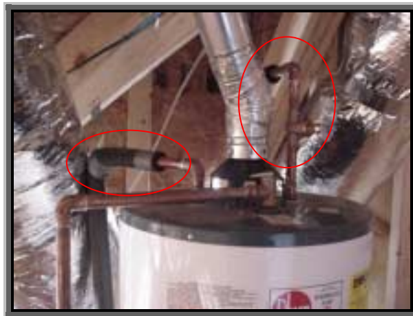
Insulation missing; insulation not correct thickness.
