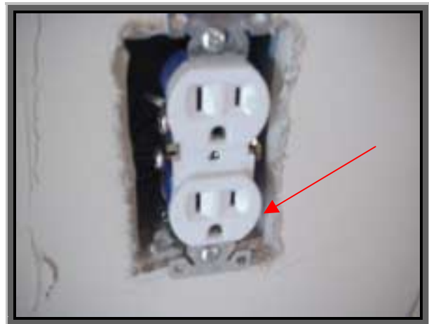
Outlet correctly sealed with durable caulking
